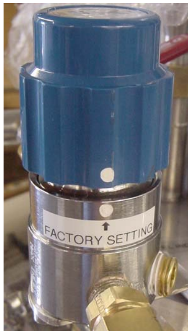
Figure 6-3: He inlet regulator marked with factory setting
