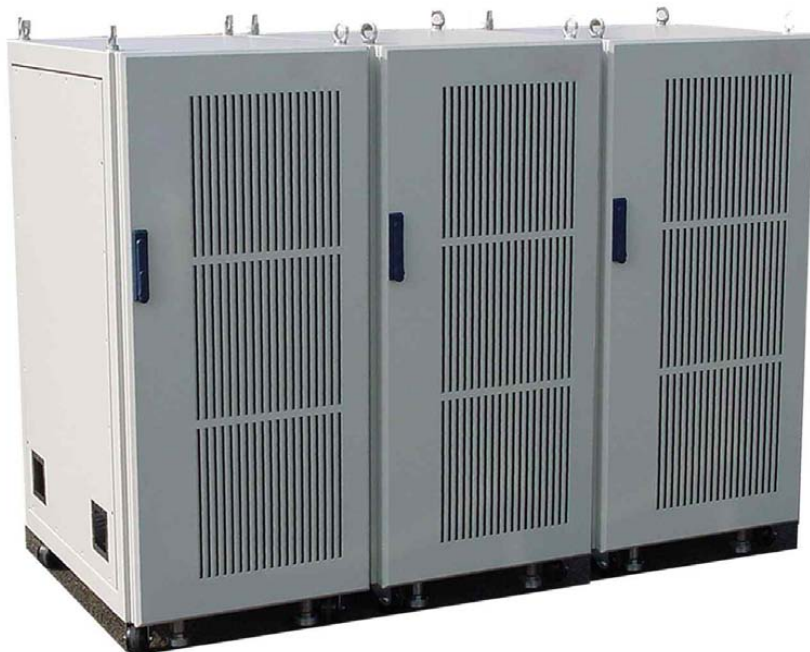
Figure 33: View of the system cabinets
