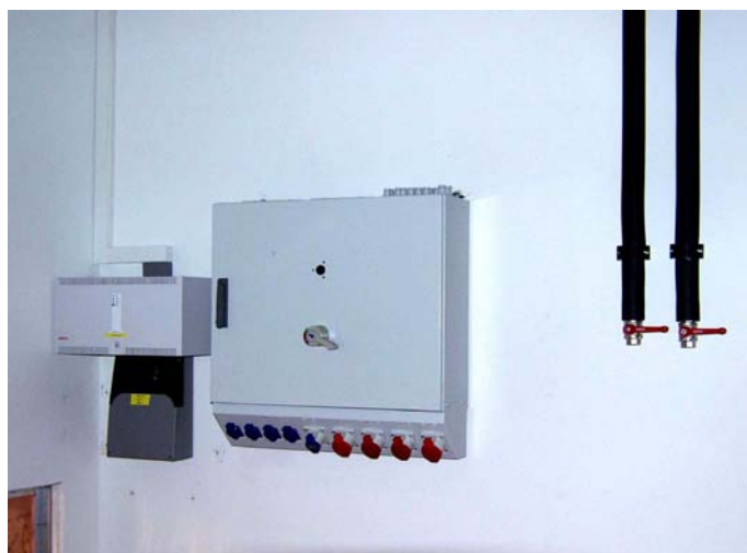
Figure 20: View of the BioSpec ® system electrical distributor and cold water connection.
