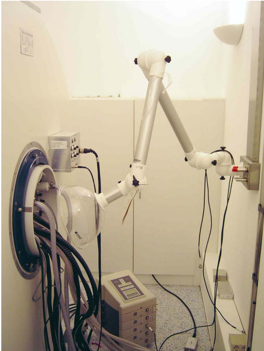
Figure 18: Example of an anesthesia gas extraction hood behind the magnet in a Faraday cage room. Model with swivel arm and extraction hood as a non-magnetic structure
