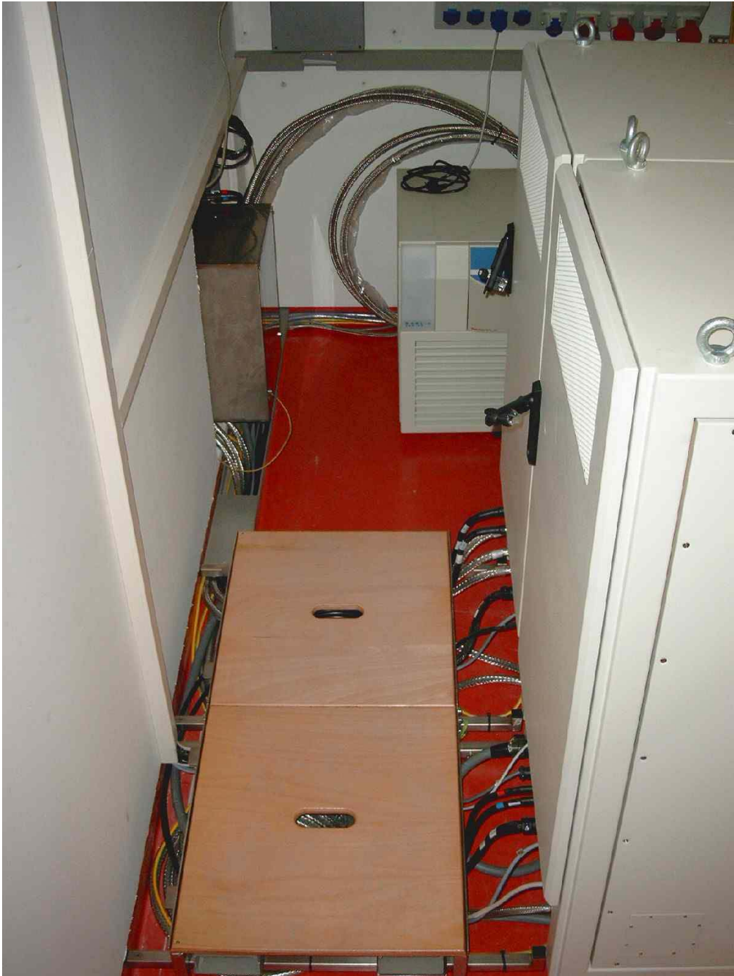
Figure 21: View of the rear side of the system cabinets and the filter plate on the left.
