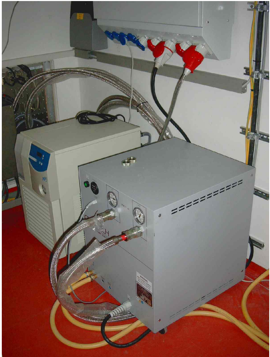
Figure 22: View of the gradient coil cooler and cryo-refrigerator. On the top you can see the connection panel of the electrical distributor.
